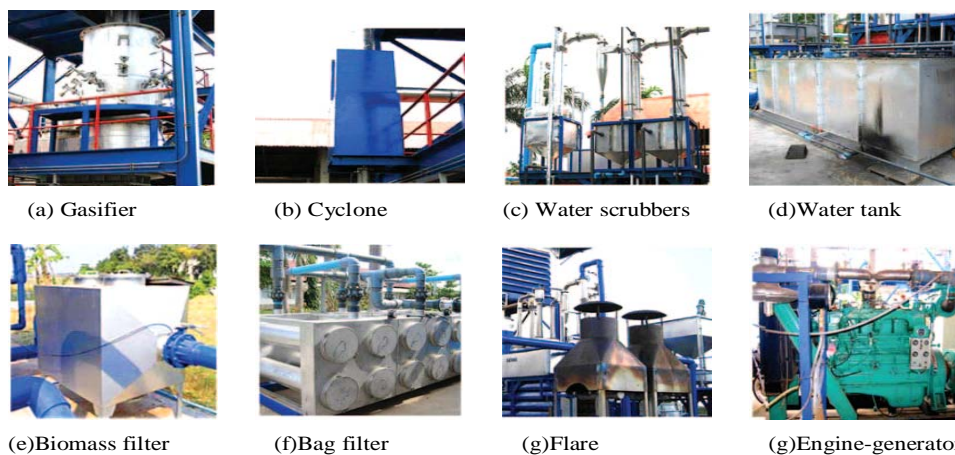
Fig. 3. The photographs of the downdraft steam co-gasification system.
