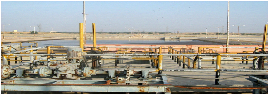
Plate 1: Huge view of jorbir wastewater treatment plant at Bikaner Rajasthan, India
