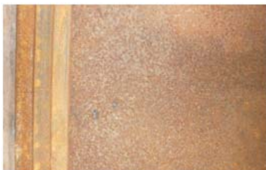
Fig. 4: View of Rusted iron sheet at 3 feet distance
