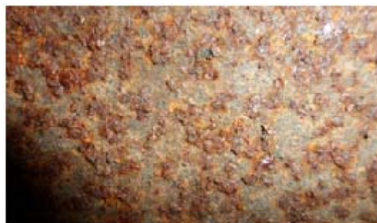
Fig. 5: Close view of Rusted iron sheet
