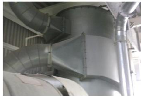
Fig. 2: Bag filter-cyclone BCIEU 24.0-37 of “Southern Rice Company”, LLC
